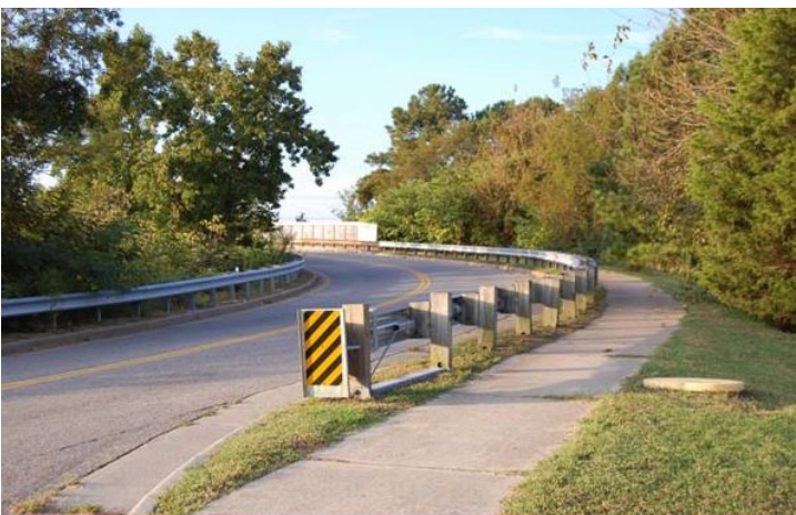
The existing bridge that connects the light rail station with Best Square is unsafe for pedestrians
