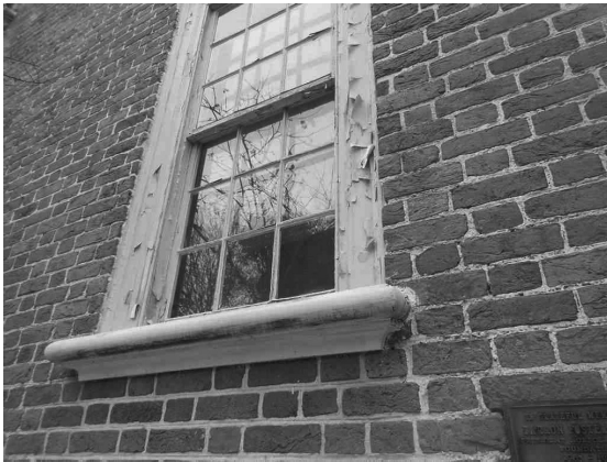
Peeling paint. Most of the exterior brickwork appears original
