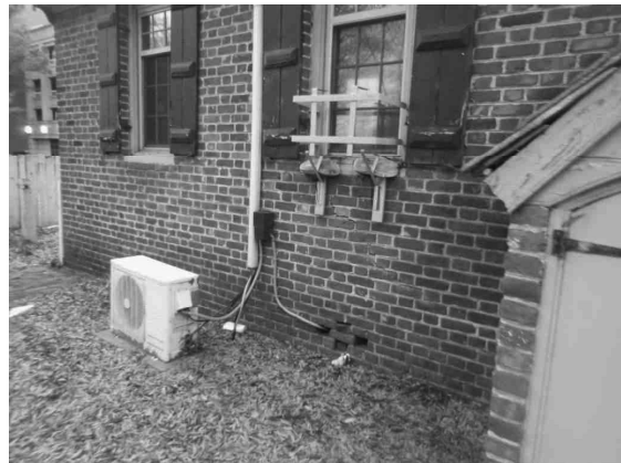
The ADU is heated and cooled by this mini-split system
