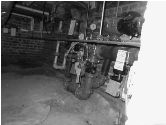
Basement is accessed through the rear shed. This is the commercial fire suppression system
