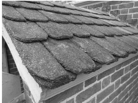
The shingles on the shed appear to be a concrete mixture
