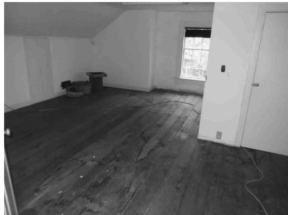
Attic - the ceiling height does not meet ANSI standards for GLA, but it could be converted to usable area
