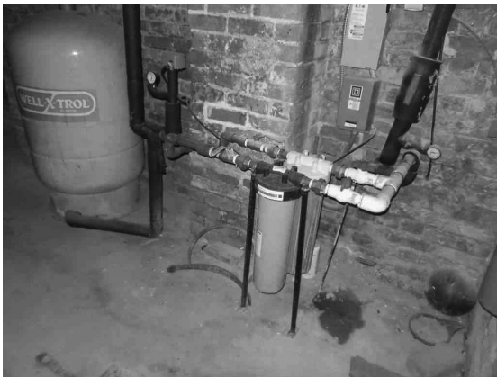
Water filtration system
