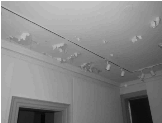
Peeling paint on most of the ceilings, but does not appear to be from water intrusion (likely from improper surface preparation)
